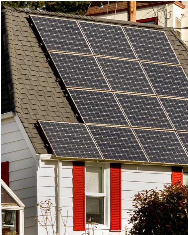
Rooftop solar panels
