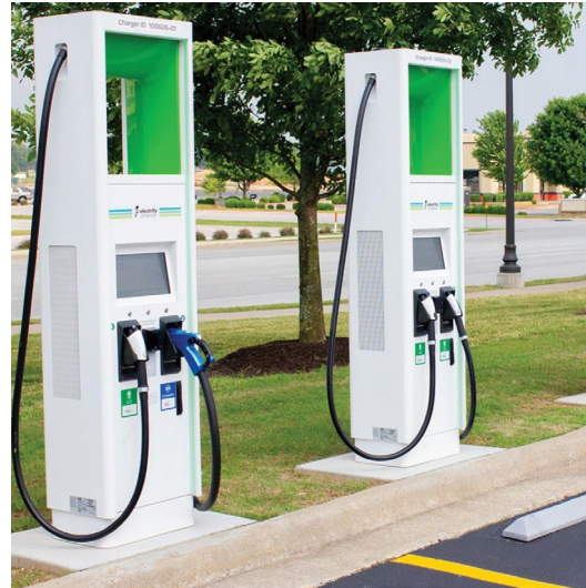
EV charge station setup
